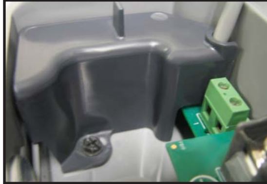
Figure 15: Plastic Cover Installed In Terminal Box
