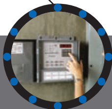
Whole home energy controls
