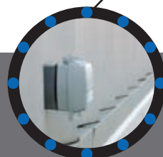
Exterior receptacle covers
