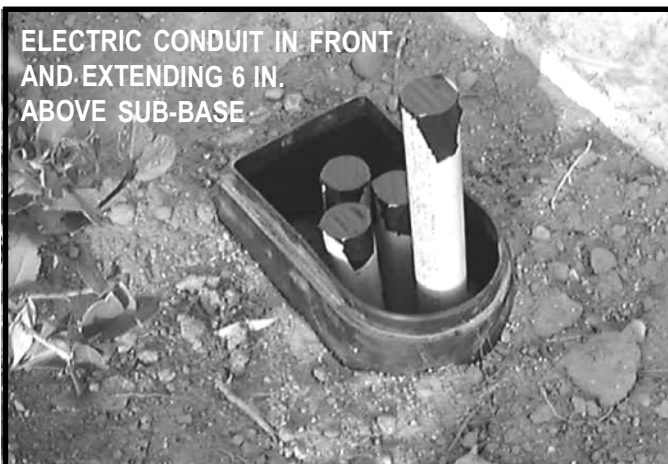
4. Backfill 1 to 4 in. below shoulder for mulch or concrete. Cut fiber conduit below or at top of base.
