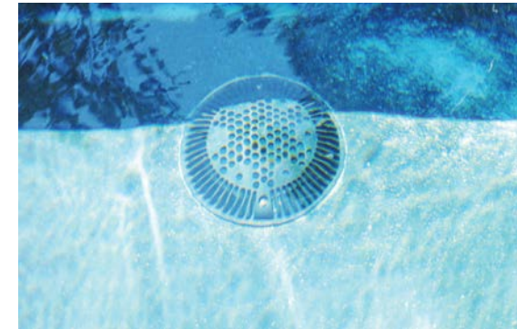
Calcium phosphate scale build up in spa drain
